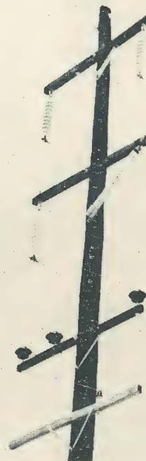
Fig. 9. Polymer Insulators in service on a 69 kv line of The Florida Power & Light Company at Juno Beach, Florida.
