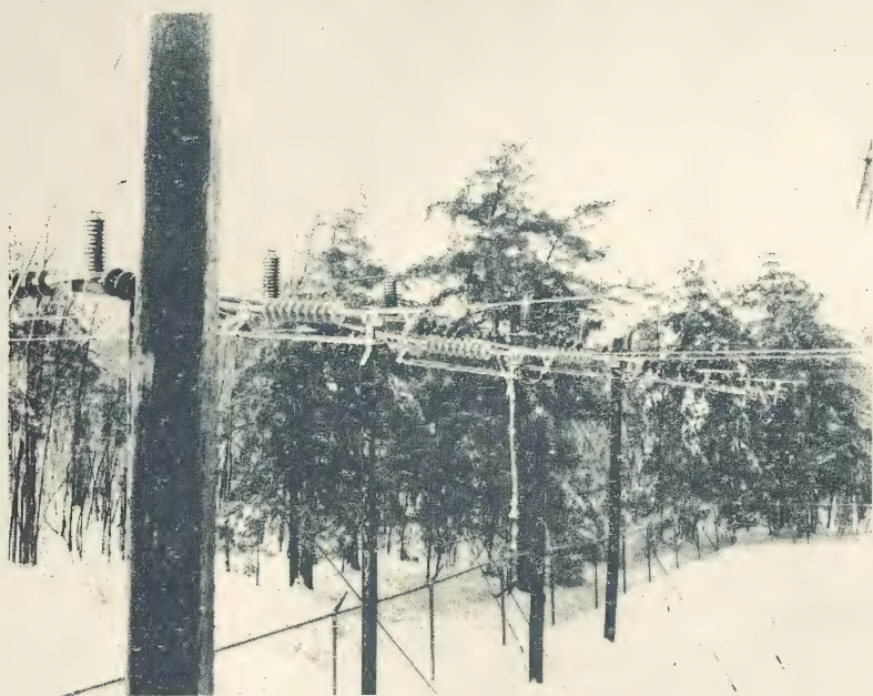
Fig. 11. A special application of Polymer Insulators on a 69 kv line of The New England Electric System.
