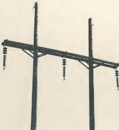
Fig. 7. Polymer Insulators in series with standard porcelain suspension insulators on a 115 kv line of The Baltimore Gas and Electric Company.
