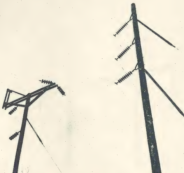
Fig. 10. Polymer Insulators in service on a 69 kv line of The New England Electric System.
