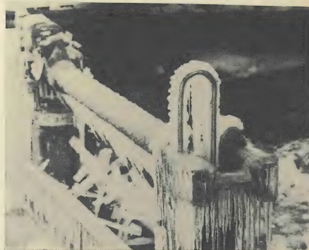
Fig. 15. Ice Test 1600 Amp. 161 KV Switch. Next Stage - Beginning of Opening Phase.
