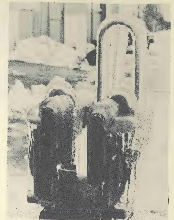
Fig. 11. Ice Test 1600 Amp. 161 KV Switch From Open to Close. First Sequence - Jaw Assembly Frozen with Blade Open.
