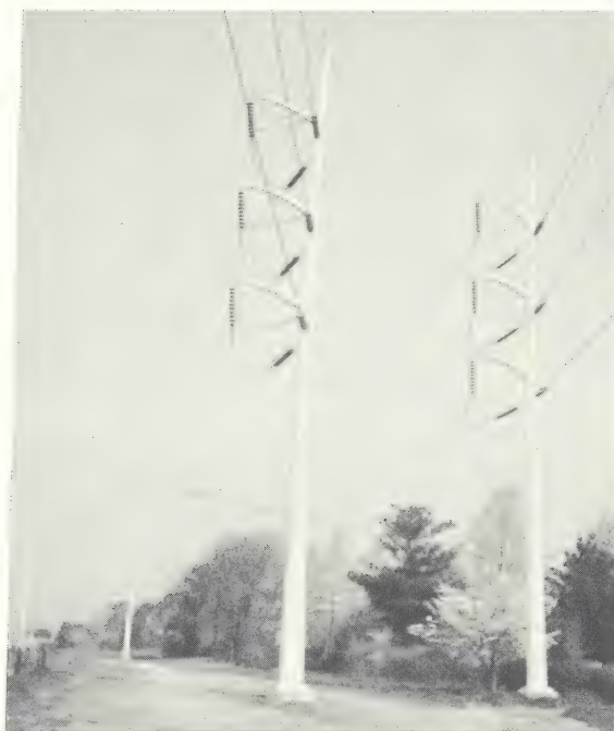
Figure IV-6. Poly-12 Steel Pole Dead-end Structure
