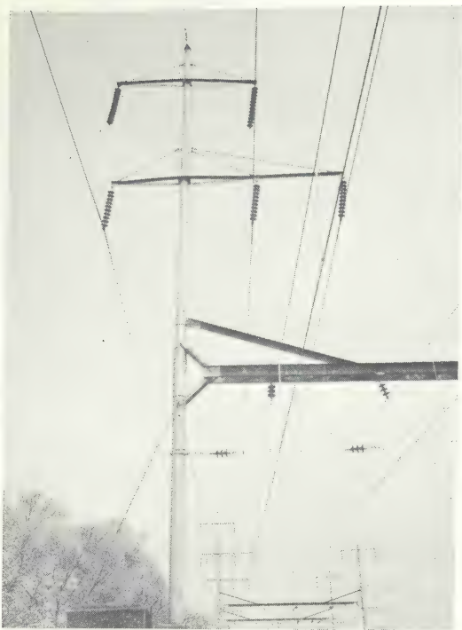
Figure IV-7. Example of 132KV Transmission Line Supported by Steel Pole. P. E. Co. Line is on Second Arm Supporting Three Conductors.
