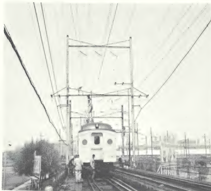
Figure IV-8. P. E. Co. 69KV Line Supported by Top Horizontal Beam. Line Located on Railroad Trestle and is Above Other Railroad Electrification.
