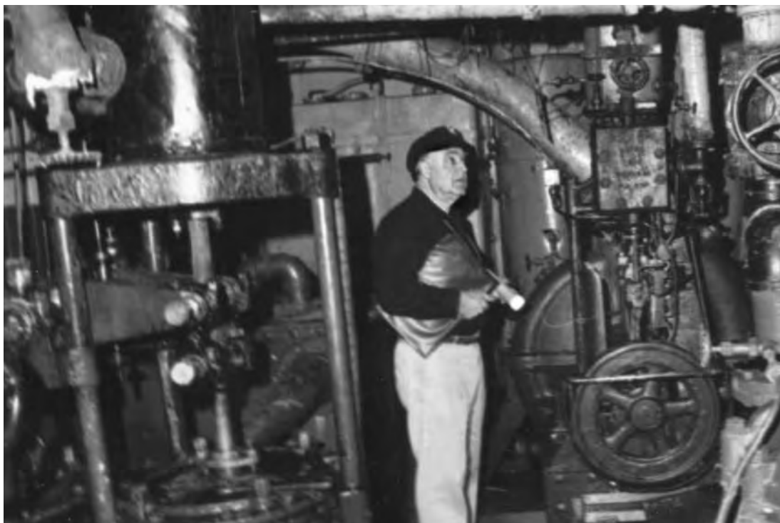
The Maritime Museum's Ken Reynard looks slightly alarmed by the grimy engine room machinery in November 1972, before she was purchased by the museum. He stands between the condensate pump and main seawater circulating pump.
