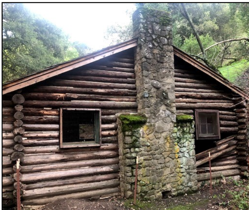
San Jose City Landmark— Pioneer Log Cabin at Alum Rock Park in disrepair.
