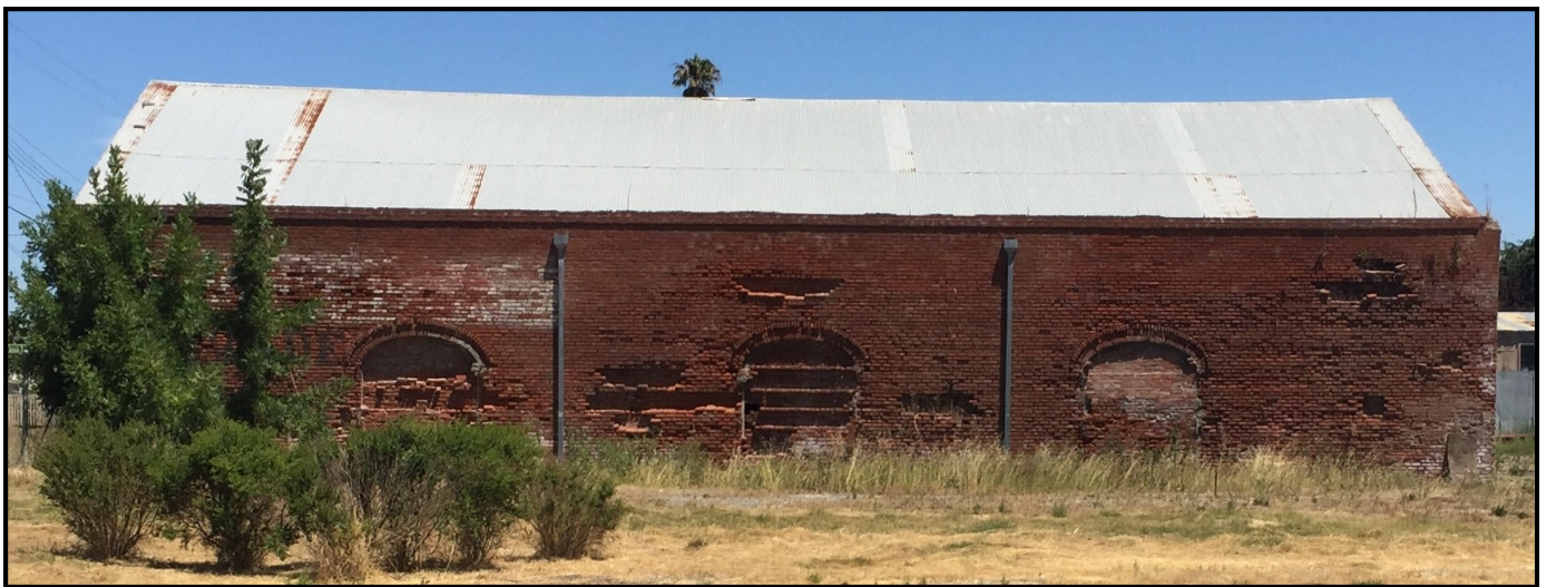
Top photo: Harry G. Wade Warehouse c. 1860s, at Alviso, a San Jose City Landmark but in extremely poor condition. Above: South side wall of the Wade Warehouse. Loose bricks and deterioration is of great concern. (Photos: Gayle Frank)
