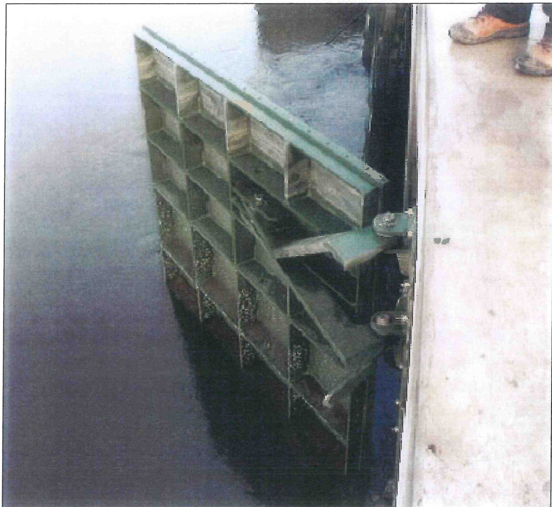
Tidegate Mounted on Concrete Vault
