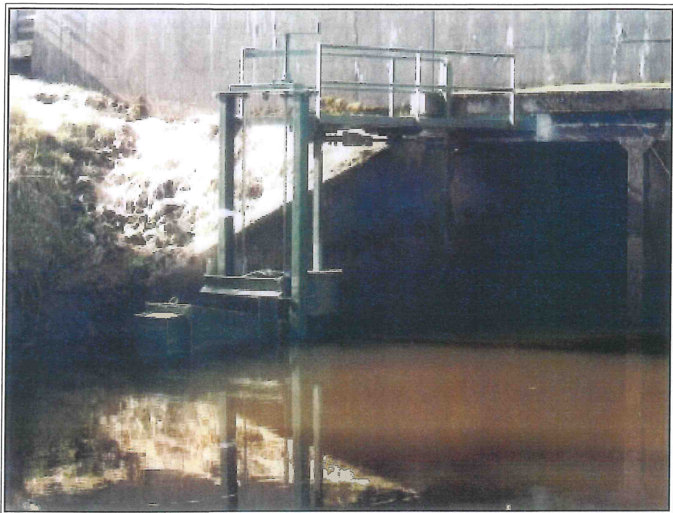
Float and Linkage Assembly Mounted on Headwall
