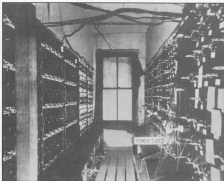
Figure 17. The rear of the first five racks on the right side, and the front of the second row on the left. The RF connecting leads can be seen overhead. The first three racks in the second row held power tubes fitted with bases.
