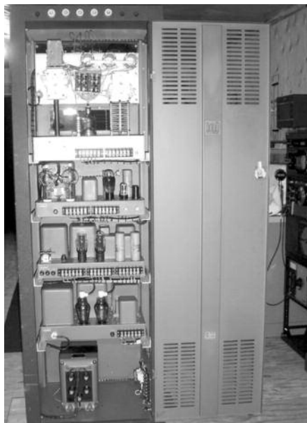
Rear view of the 30K-1 with access door open. From the bottom: plate transformer, high-voltage supply, low-voltage supply, modulator, final, and output network.
