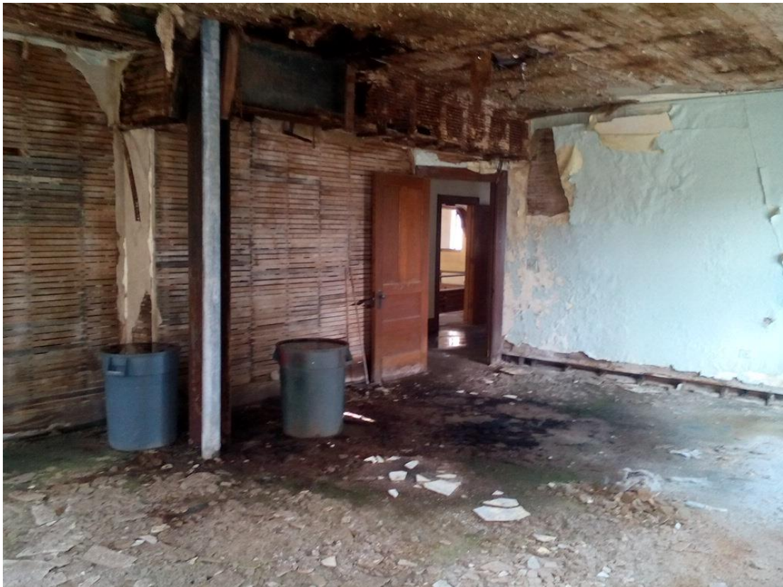
Condition of many upper rooms due to roof leaks and holes.
