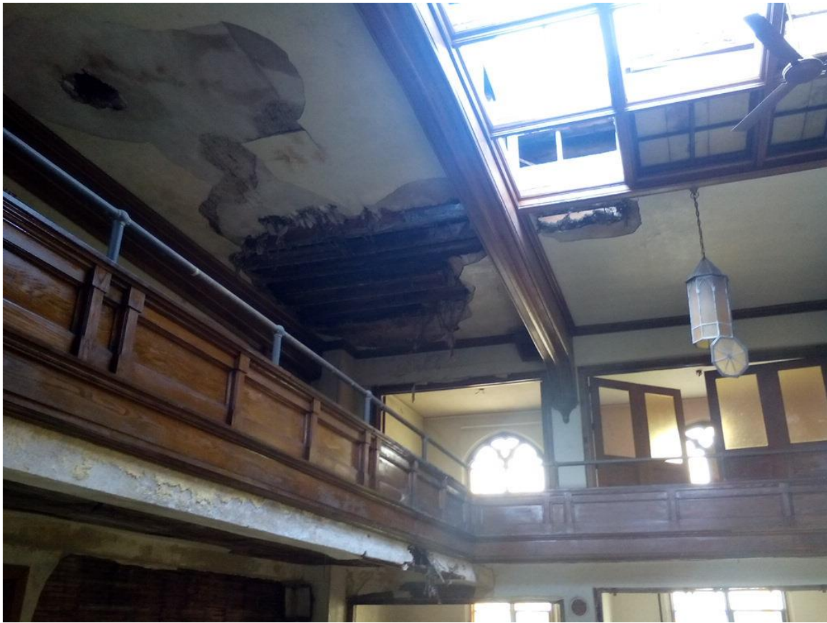
Auditorium skylight and ceiling damage.
