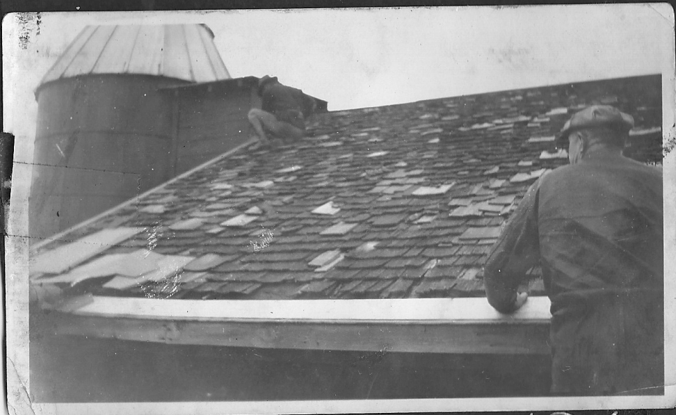
Stewart Teator Arthur Bathrick barn roof
