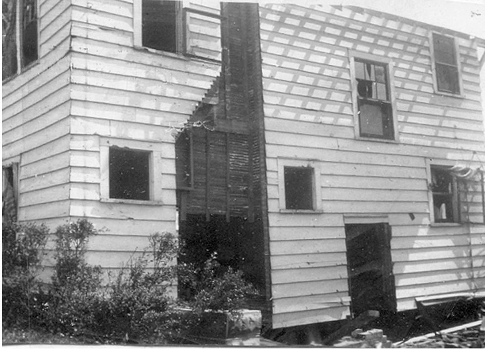
The South side of the house shows how far it had moved and the debris in the basement.
